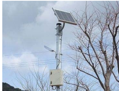
LED防災防犯灯
